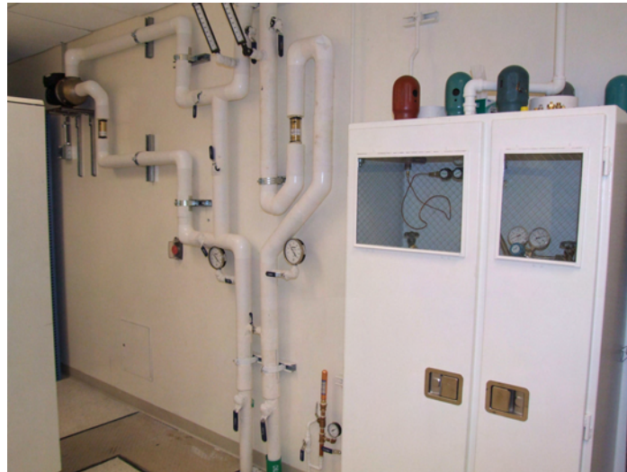
Building chilled water supply. Since flow is only 3-4 gpm, a separate booster pump was installed (upper left corner).
